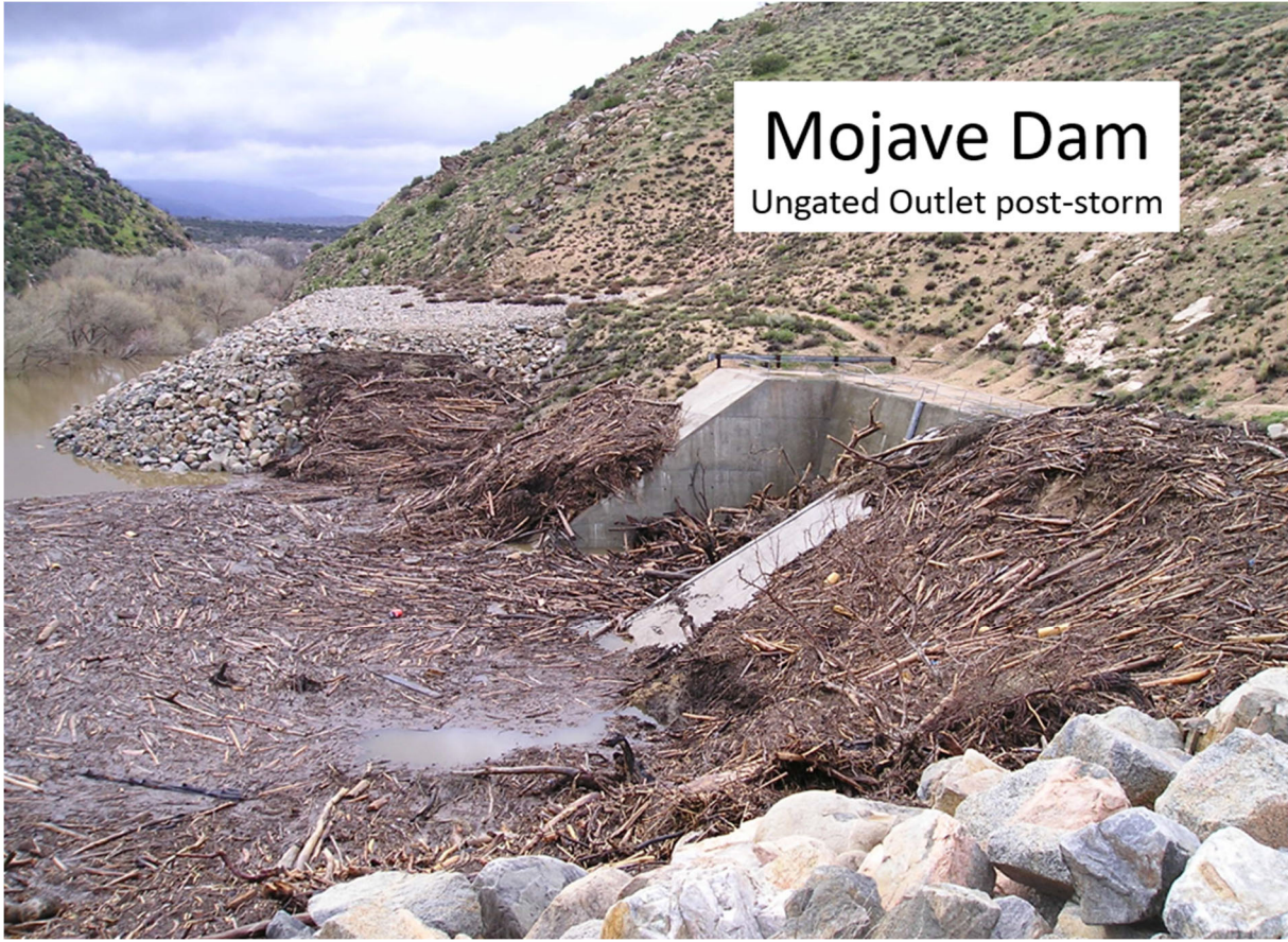
Figure 15. Mojave Dam outlet post-storm (upstream end of outlet; USACE photo).
