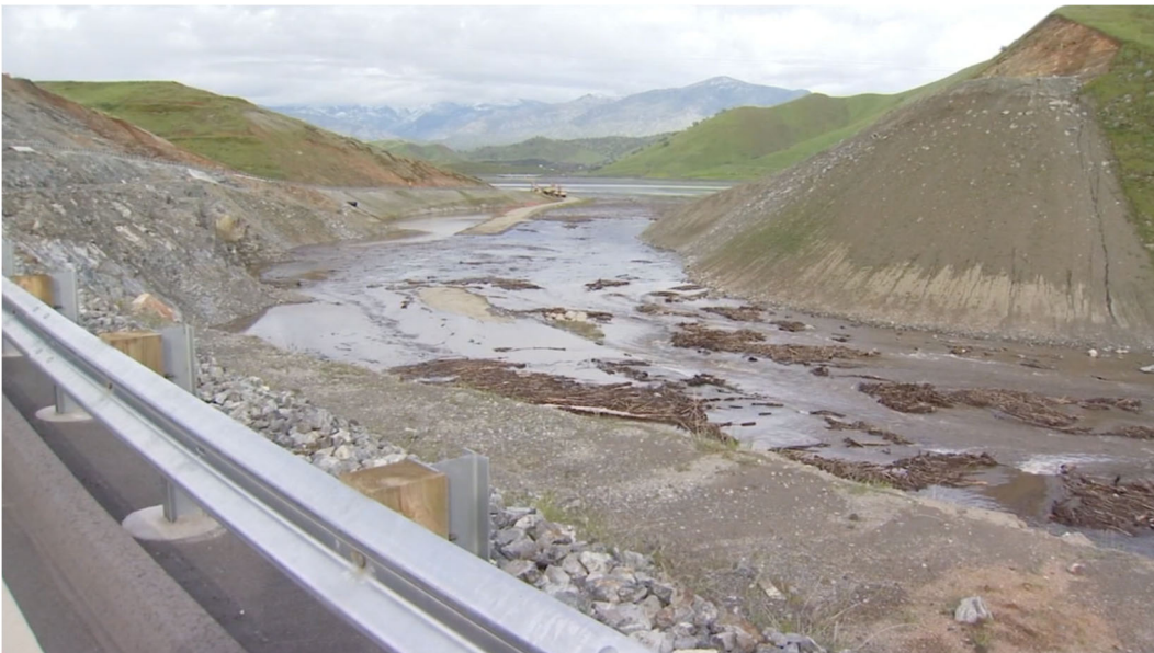
Figure 32. Debris piles below Schafer Dam after a high flow event (USACE photo).
